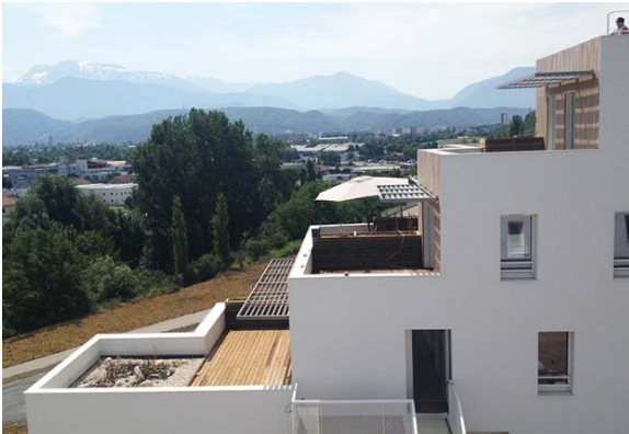
Fig.8. Extensive green roof after plantation
